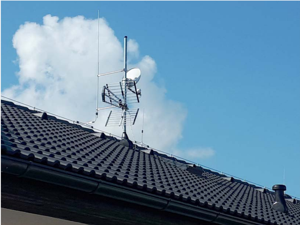
Fig. 9 Example of a properly arranged receiving antenna system installed on a family house (using principles shown in Fig. 2).
